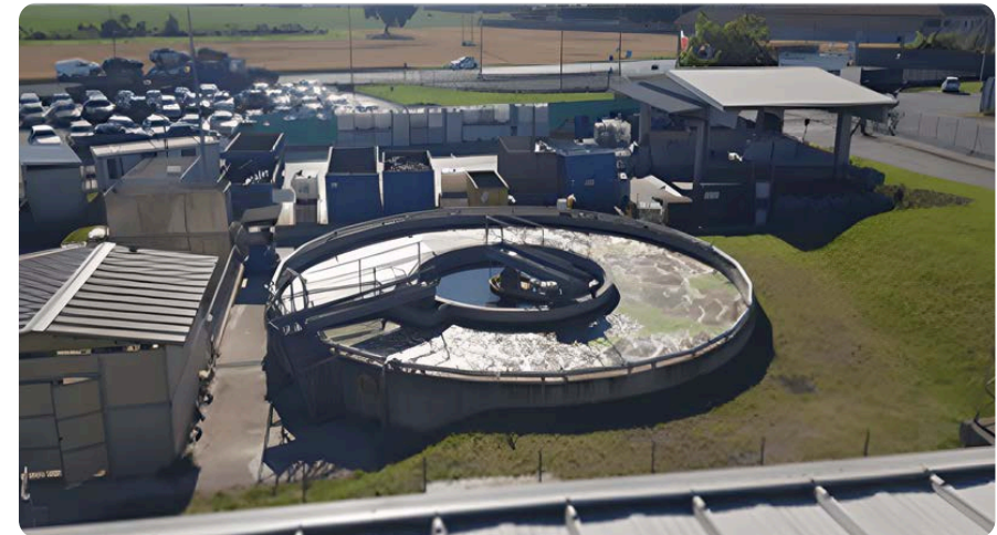
Water treatment equipment in CIR plant
